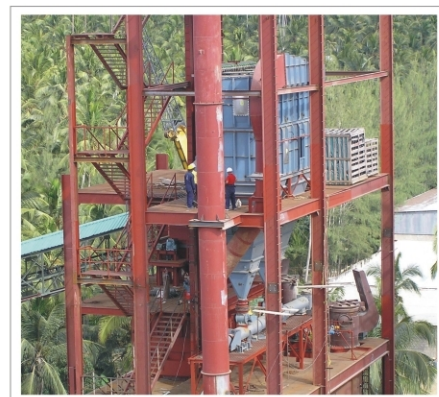
COAL MILL BAGFILTER
