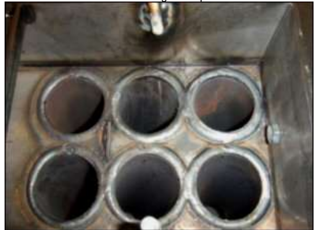
The tubes shown on this picture without the flue gas break that you can see on the picture to the left.
