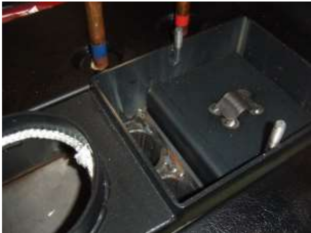
Under the door on the top of the boiler, you can reach the tubes at the regular cleaning of the heating surfaces
